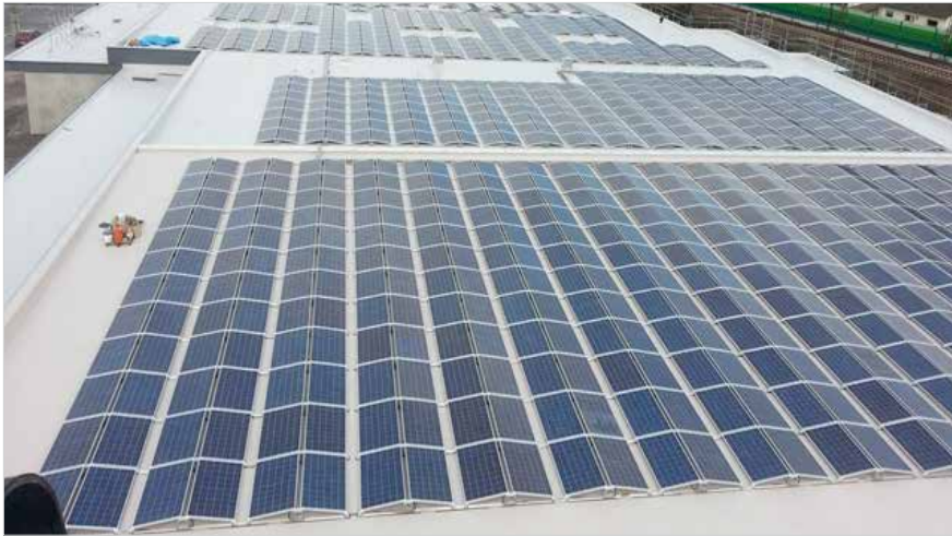
Hemsbach | Germany Installation: 350 kW | D-Dome System
